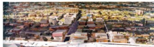
Construction site for the highway in Cambridge, showing the area where the inner belt is being built.
